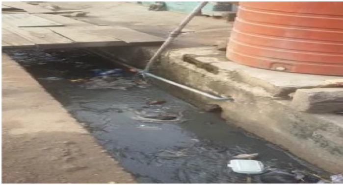
Plate 1: water pipe in open drains
